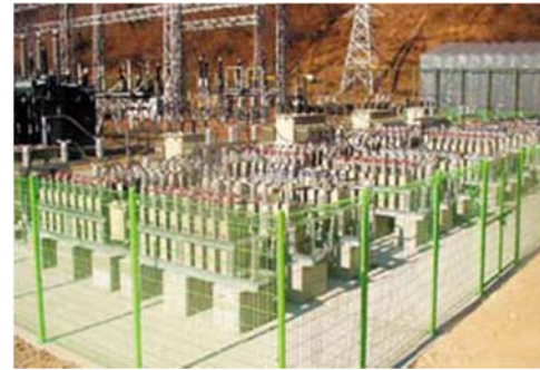
Harmonic Filter Bank 22.9kV 63Mvar
