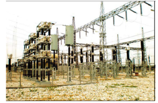
Capacitor Bank 150kV 25Mvar for substation
